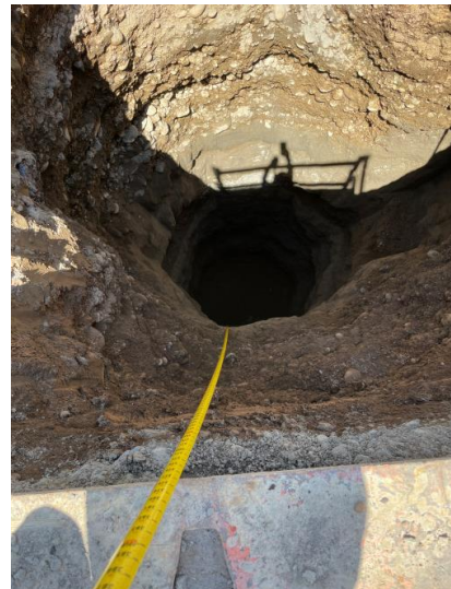
The excavation – 31 feet deep and 9.5 feet in diameter – shown from the “observation area”
