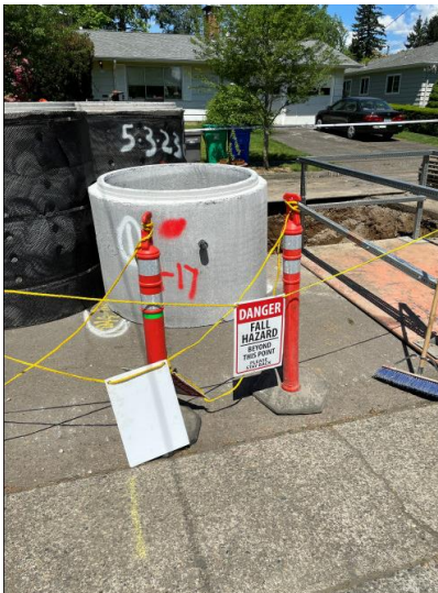
A concrete block the company used to anchor the fall-restraint system
