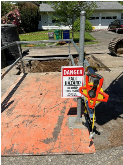
The “observation area” that employees used to guide a precast chamber into the excavation
