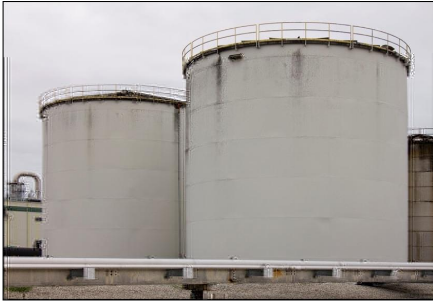
Figure II.15 Product Storage Tank
