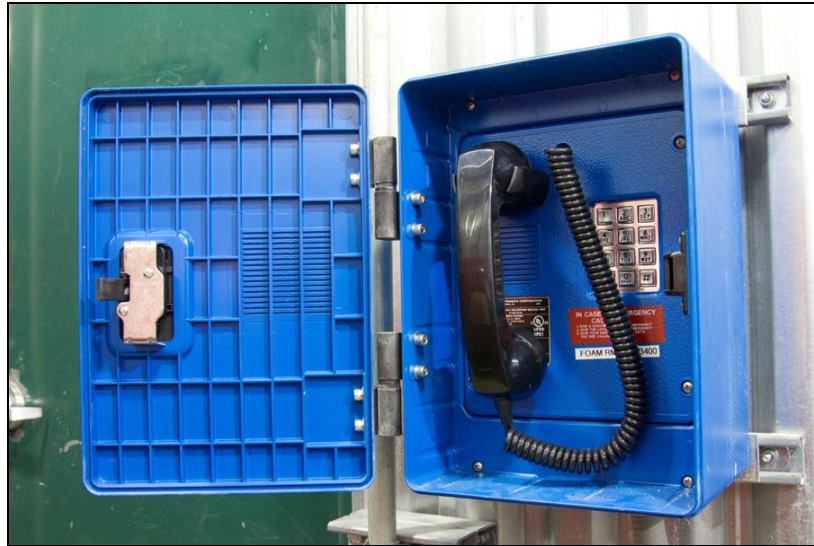
Figure IV. 1 A Telephone Rated for Class I Hazardous Locations
