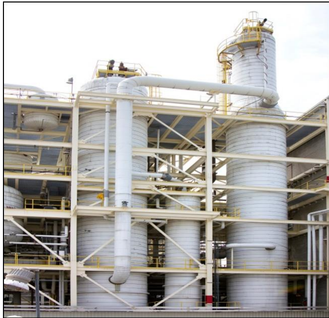
Figure II.13 Ethanol Distillation Columns
