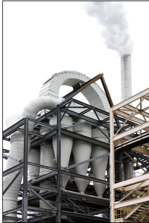
Solids Recovery Cyclone
