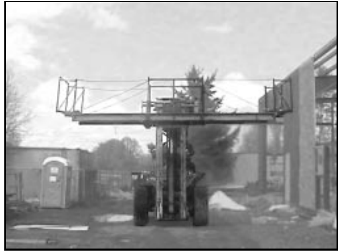
AMSE/ANSI Standard B56.6-2002 [8.24.1(b)] says a work platform floor can't exceed the overall width of a rough-terrain lift truck measured across the load-bearing tires plus 10 inches on either side. The platform on this truck exceeds the overall width of the truck by a substantial margin.
