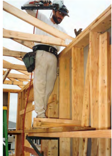
Interior scaffold brackets designed by the home builder.
