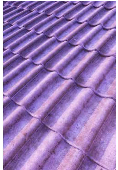
Old purple corrugated asbestos cement roof sheet.
