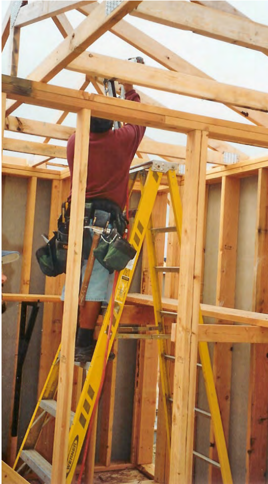
Working at the peak from the top plate of an interior wall.
