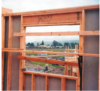
Make sure door and window openings are properly guarded.
