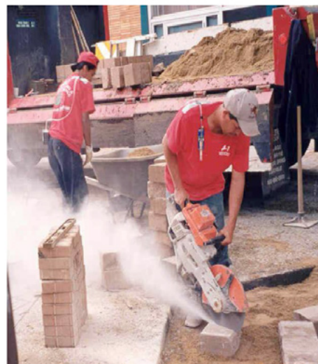
Without dust controls, using a handheld power saw to cut concrete can expose workers to high levels of respirable crystalline silica.
