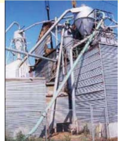
The top of the factory roof was destroyed in the wood-dust explosion. — Oregon
