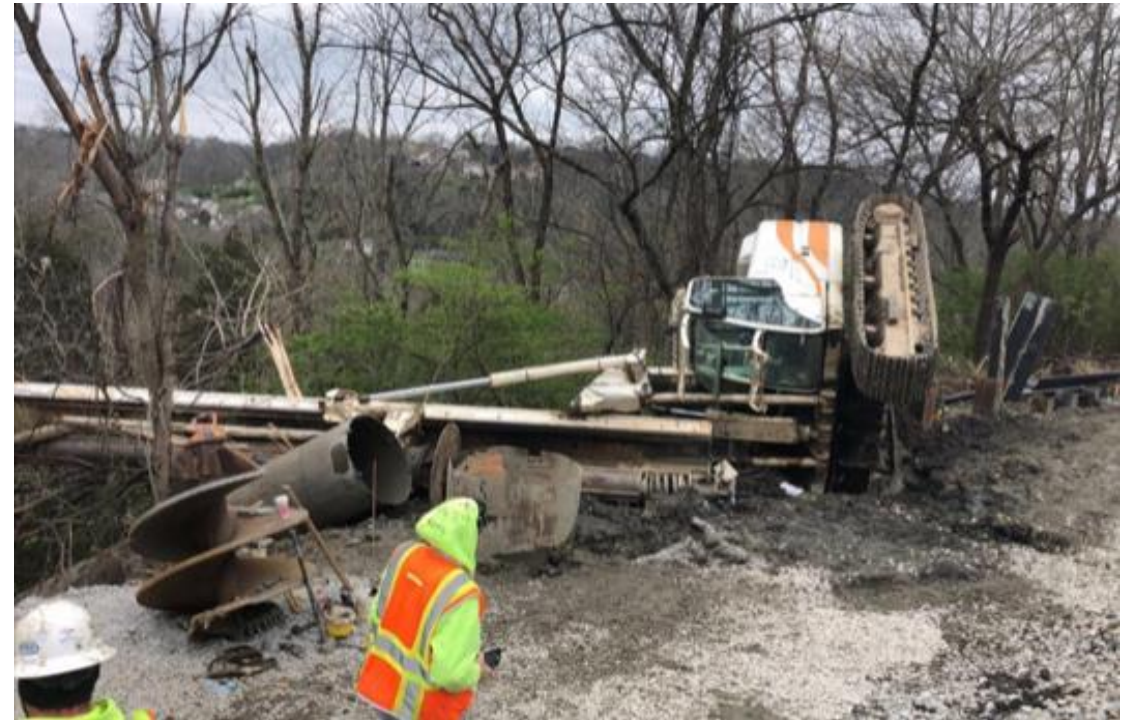
Unsafe ground conditions for equipment
