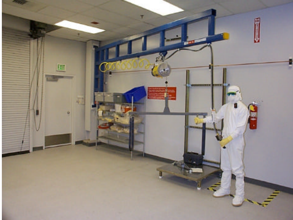
Crane installed to assist maintenance technicians in lifting heater cores
