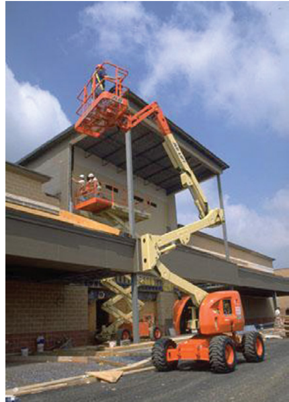
If you work from an aerial lift, you must be protected from falling.
