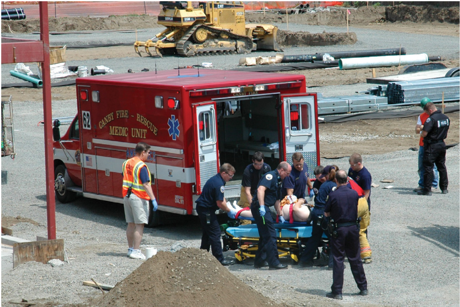
Paramedics treat a worker who fell 25 feet through a hole on the roof of a construction project.
