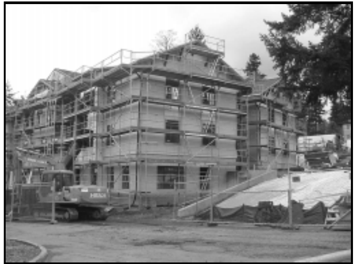
One of the three new buildings that make up the Campus Housing Project at Lewis & Clark College in Portland.
